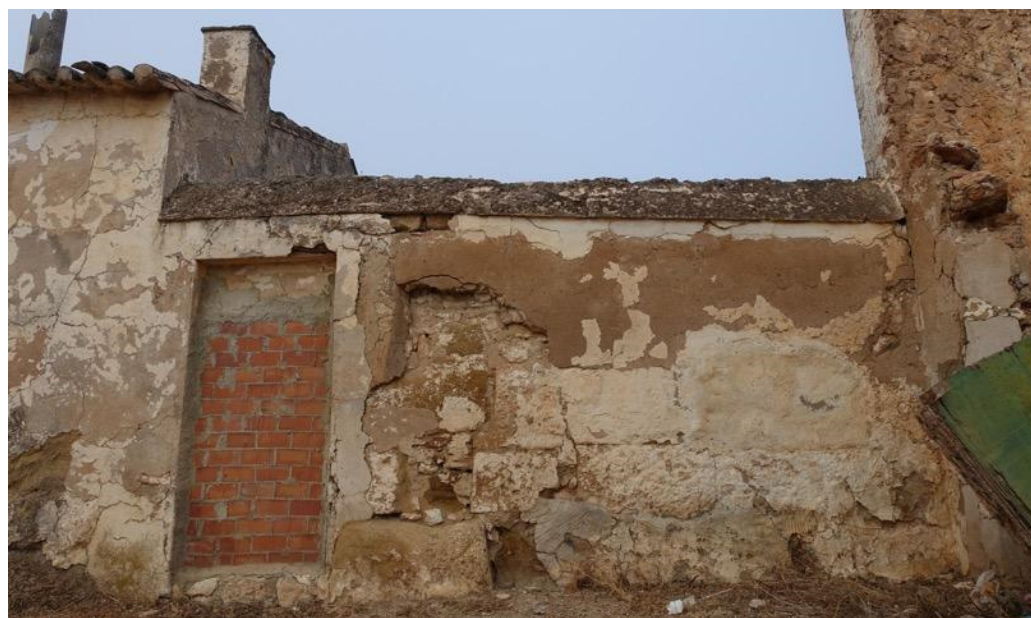
Figure 15. Remains of the jamb of the doorway that opened onto the central courtyard (Phase 3, A102, SU1050, 1051); change in masonry technique (Phase 3, A103, SU1052), right; and collapse of the doorway (Phase 4, A111, SU1053). For stratigraphic sequence see Figure A4.
