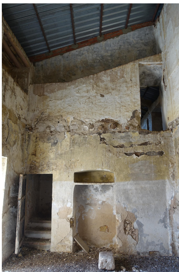
Figure 20. Partition wall (Phase 6, A112) separating the eastern and western sections of the original hall, upper storey added (Phase 6, A113), and blocking of the northern opening (Phase 6, A113, SU1095).
