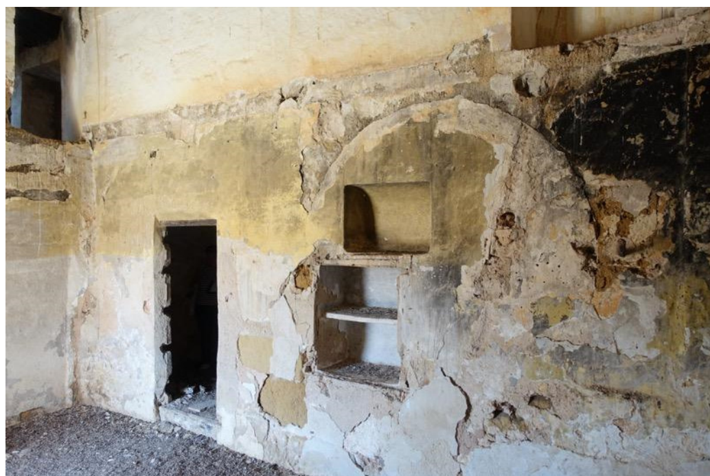
Figure 12. Section of the interior arcade preserved in the southeast house (Phase 3, A102, SU1089) and remains of the alfiz at the junction with the later perpendicular wall (Phase 6, A112, SU1097, 110).
