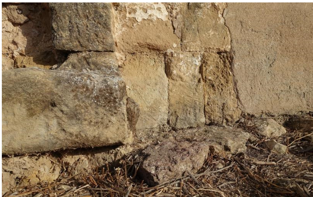
Figure 18. Blocks belonging to the preserved pavement in the corner of the northwest arcade (Phase 3, A105, SU1076) and detail of the ashlar masonry. For stratigraphic sequence see Figure A7.
