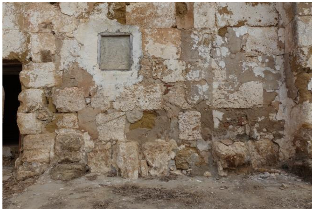
Figure 6. Lower course (A101, SU1012) and elevation of the southeast front (A102, SU1001) of the main hall (Stage 3). Window put in later (Stage 6, A128, SU1015). For stratigraphic sequence see Figure A1.
