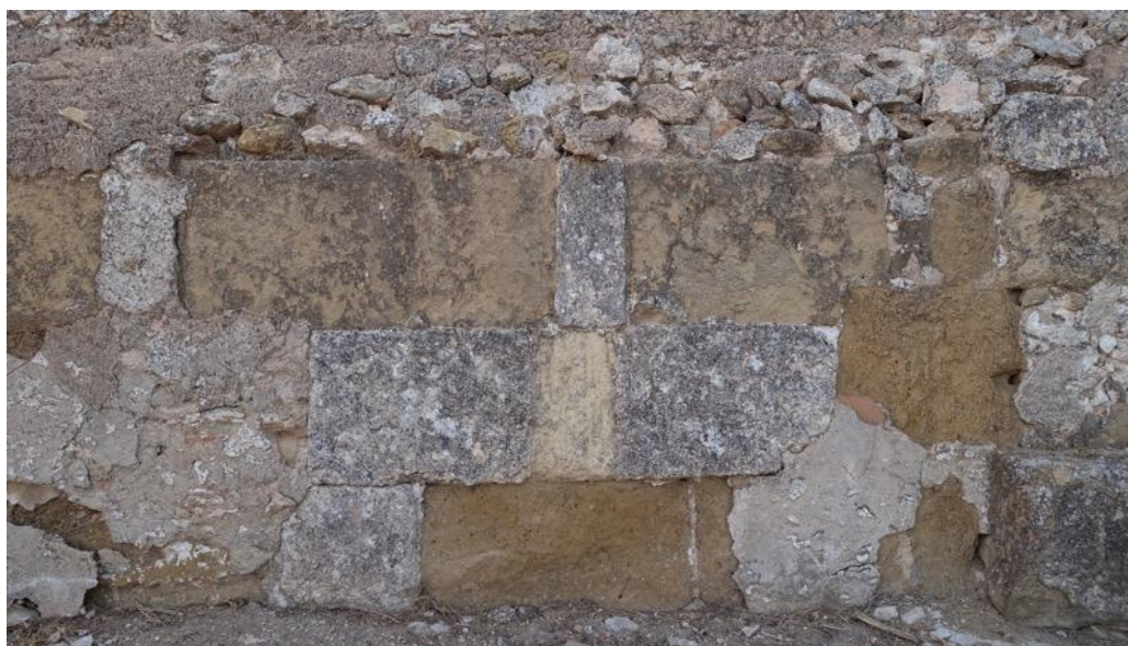
Figure 16. Interior of the northeast façade: regular masonry of stretchers and headers on the left (A103, SU1052) and junction with the earlier masonry on the right (A102, SU1051). For stratigraphic sequence see Figure A8.
