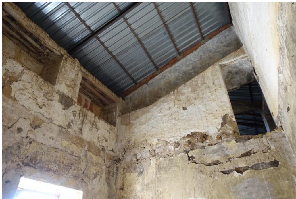
Figure 21. South corner of the second-floor elevation of the southeast house (Phase 6, A113).
